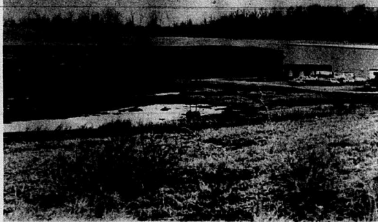
Before the snow came, this picture was taken of clearing and excavation that has started at Mt. Vernon Plastics where an additional building is to be
