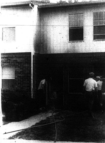
Apartment ruined by fire Lora Lee Duncan's apartment in Valley View was destroyed by fire last Wednesday, Aug. 16. Firemen say they believe the fire began in a couch, and smoke was pouring from the space when they arrive. Duncan and her three children lived there. All their belongings were lost. A workman at a nearby construction, Don Swisshelm, is credited with keeping the fire from spreading by using a garden hose to spray the fire until firemen arrived.
