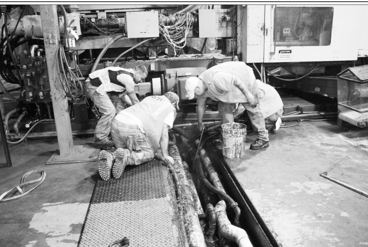
Rockcastle County Detention Center inmates on work release are shown above power washing sludge out of the trenches Tuesday afternoon at the old Plasticware factory in the Rockcastle County Industrial Park. Safety-Kleen, a waste management cleaning company from Lexington, vaccummed up the sludge. The factory is being cleaned up by work, primarily by release inmates, before Anchor begins operation sometime in May.
